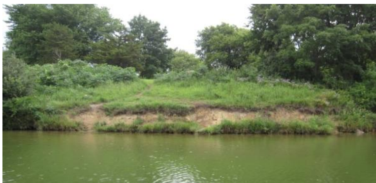
Figure 25. An example of shoreline erosion along Don Williams Lake.
